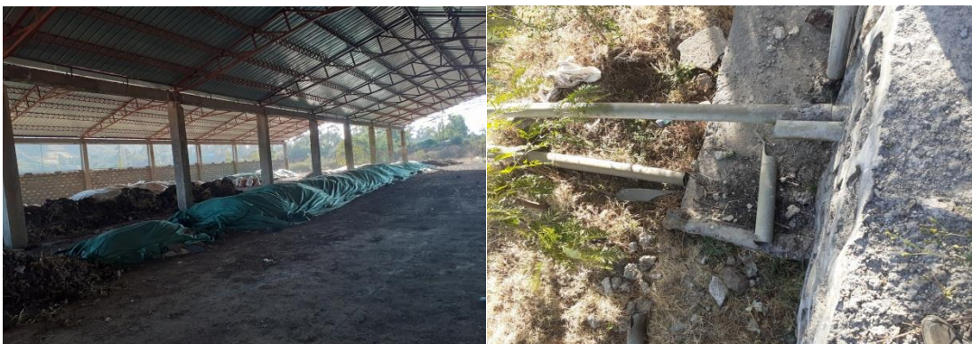
Figure 14: COMPOST shed and its damaged leachate pipes at Bishoftu
